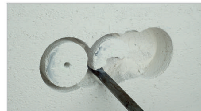
4. Level out the space using a chisel and adapt it to the shape of the junction box.
