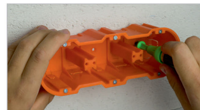
2. Mark central points with the use of marking openings in the bottom of the junction box.
